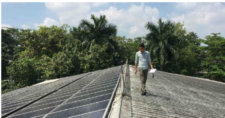
An electrical engineer from SMART Myanmar evaluates an 80 kW solar PV system at a garment factory in Yangon in Nov., 2018.
