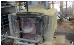
Old Inefficient Boiler
