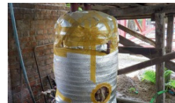
Old Condensate Recovery System
