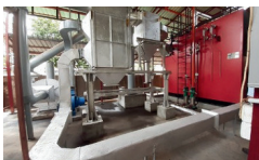
Newly Improved Boiler
