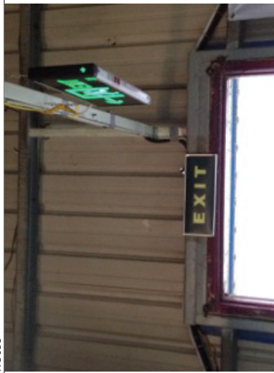
No emergency light installed
