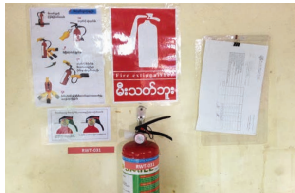
Fire extinguisher including information for usage
