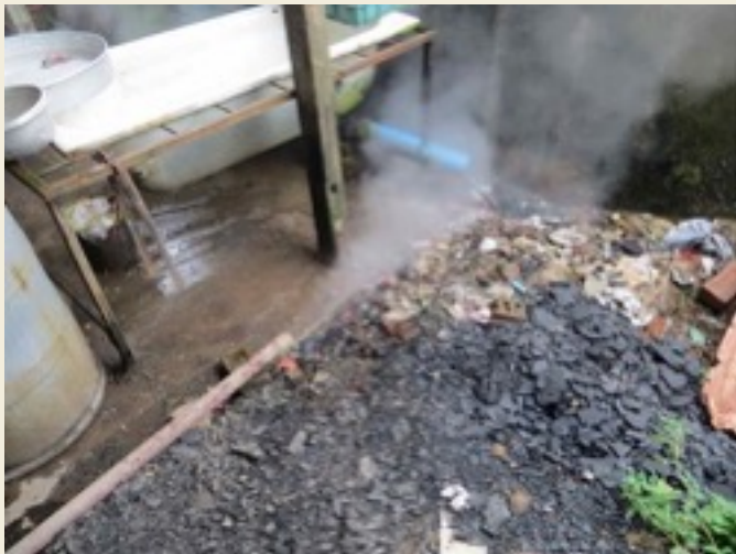
Condensates drain releasing too much steam
