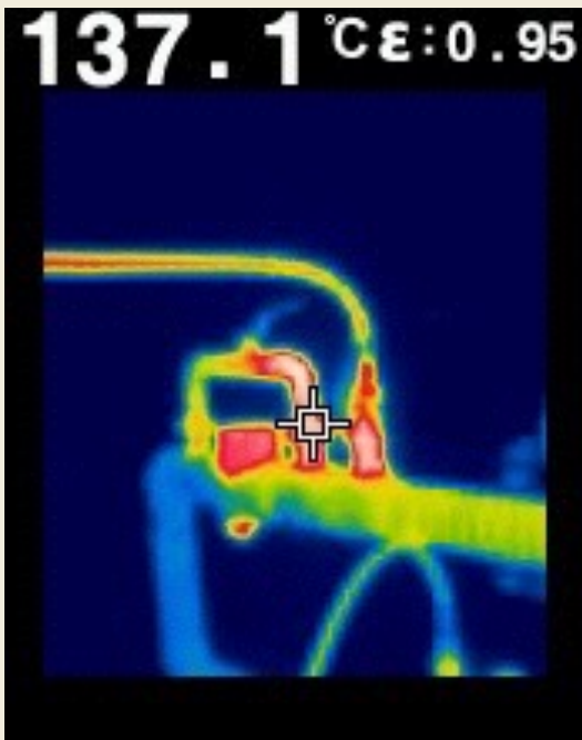
Steam piping network at factory C
